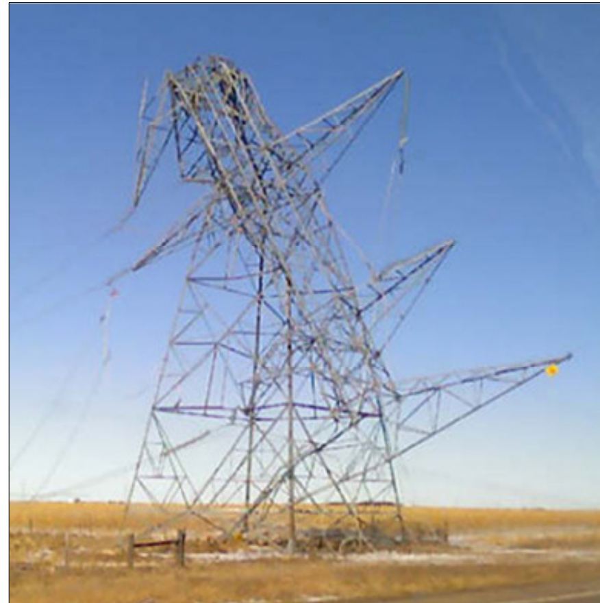
Late December ice storms crippled this 345kV line near Axtell, Nebraska
